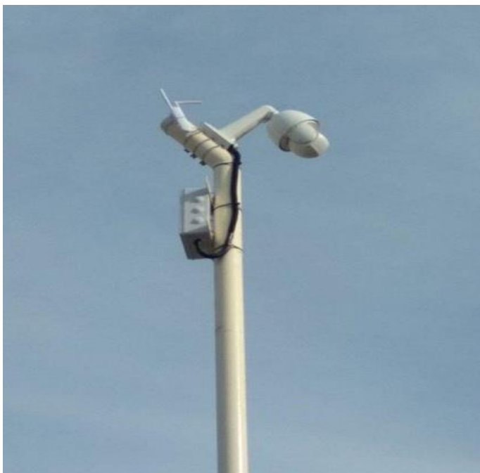
Figure 7. 4: Camera set installed on freestanding mast
