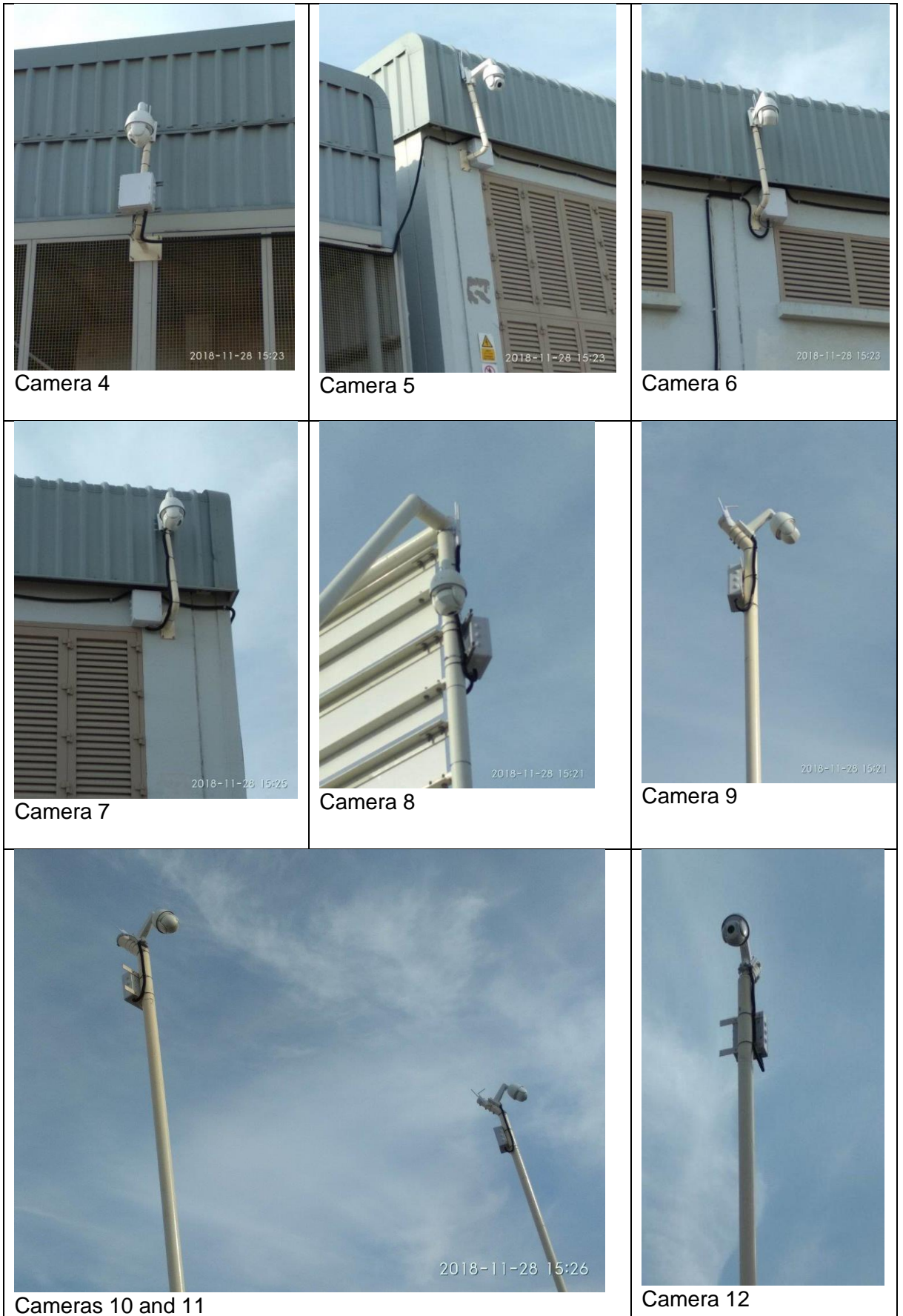
Figure 8.9: The installed 12 cameras
