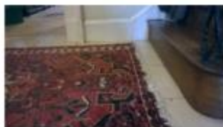
Concrete floors (put in during post-flood renovations) finished with natural limestone tiles.
