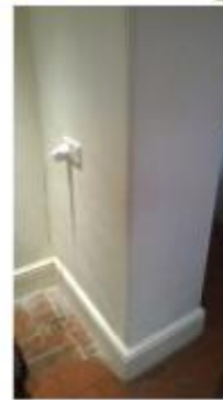
Walls - hydraulic lime plaster (with salt resistant additive) on steel mesh supported by wooden battens (to create air gap).
