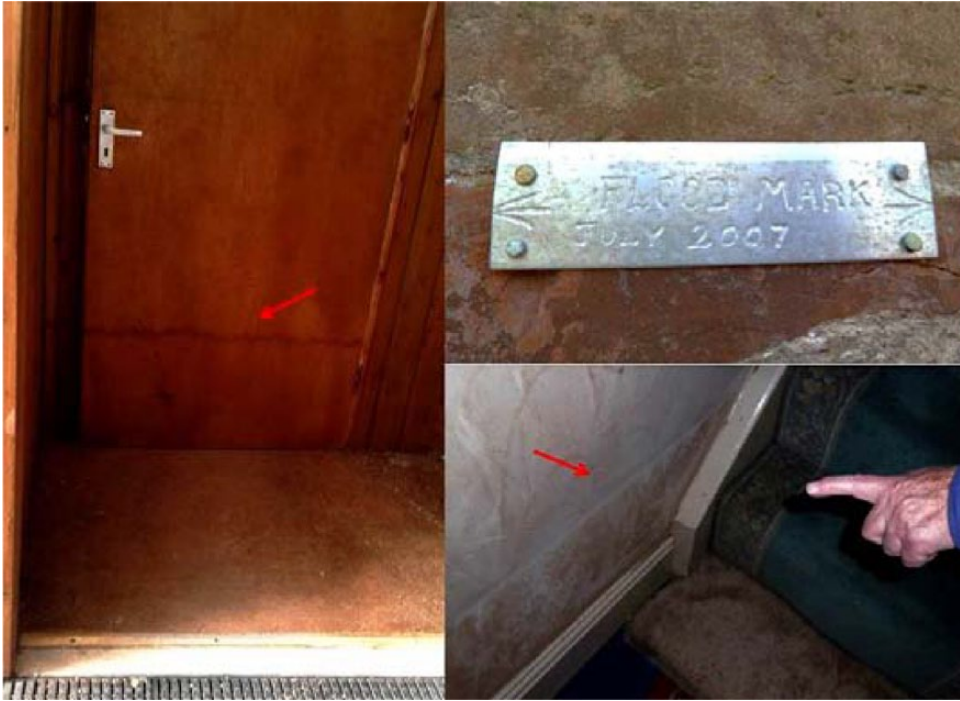
Figure 4. Unofficial flood marks of residents inside and outside their homes and gardens. Source: Andrew Holmes and Lindsey McEwen. Published with permission.
