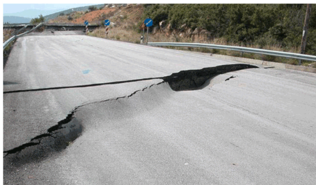
Fig. 2. Road pavement defect (U.S. Department of Transport).
