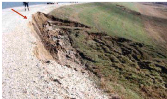
Fig. 5. Slope failure of embankment caused by expansive soil (Jalal et al., 2020).
