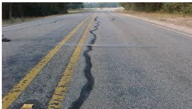
Fig. 3. Typical longitudinal crack developed on pavements over expansive clays (Zornberg and Gupta, 2015).
