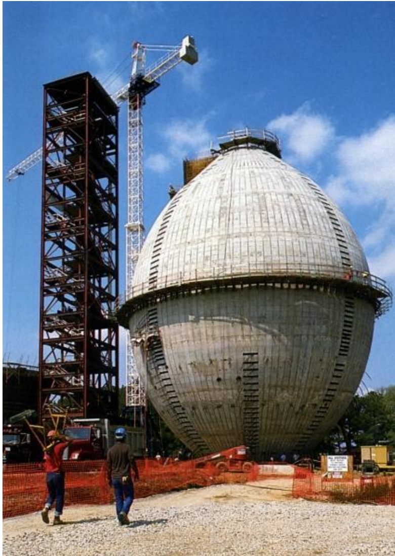
Figure 5. Prestressed Concrete QSD under construction Back River Wastewater Treatment Plant Baltimore, Maryland, USA. (Photograph courtesy Crom Corporation).
