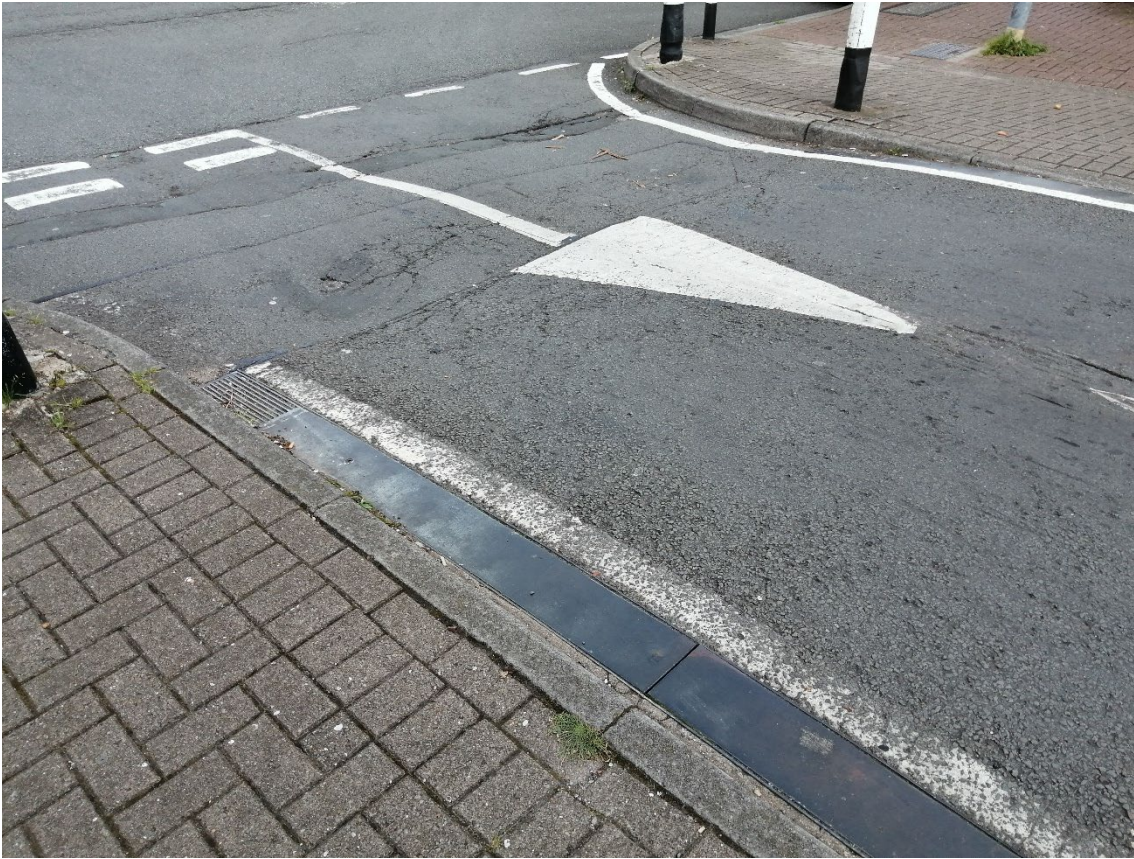
Figure 55: Kinsey Street, speed bump with markings where vehicles have hit / scraped the ground generating noise
