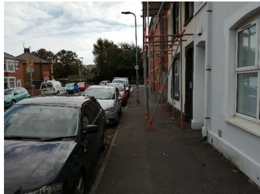
Kinsey Street, note scaffold restricts pavement width.
