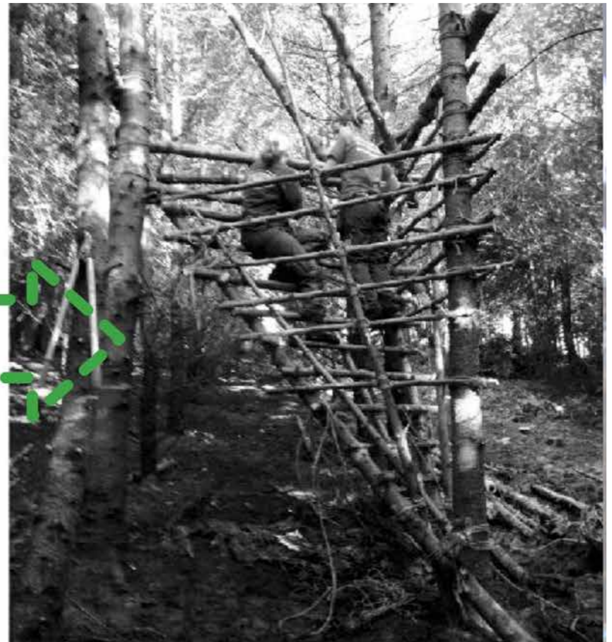
20 Left: Getting Started - initial tier, showing form beginning to be generated by process of construction
