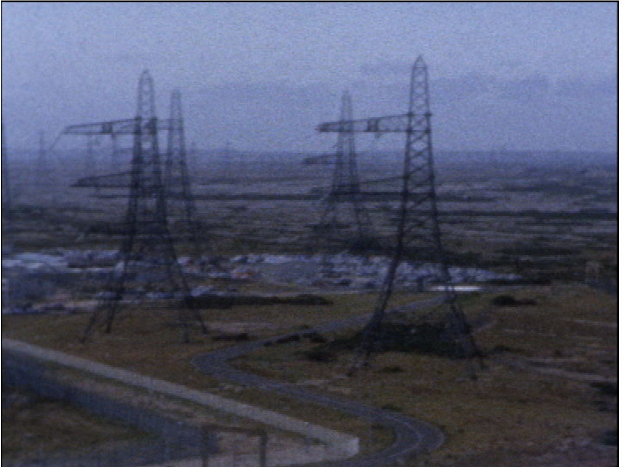
Figure 11: Pylons at Dungeness, Super 8 frame 2009
