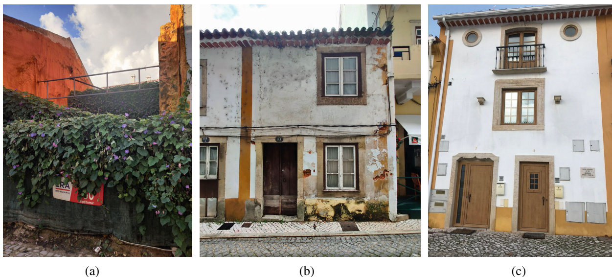
FIGURE 4 State of conservation (a) fully demolished, (b) bad state of conservation, and (c) good state of conservation.
