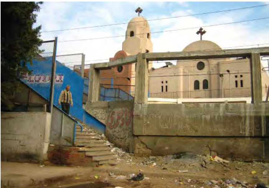
FIGURE 71. Dilapidated pedestrian bridge over the metro line in front of Coptic Cairo
