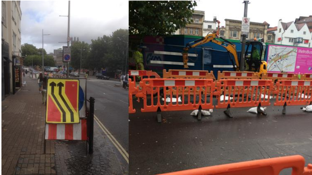
Figure 6-7: Construction works and related signs disturb the pedestrian
