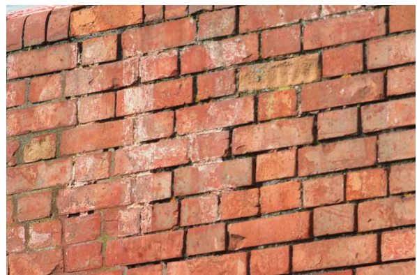
Figure 7: Eroding paintwork –you can just make out the letter ‘R’ of ‘Picture House’.
