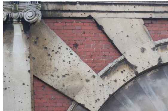
Figure 4: Detail of shrapnel damage from WWII bomb, which exploded outside the Curzon, 4 Jan 1941.
