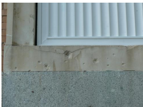
Figure 1. Shrapnel damage in the School of Medicine
