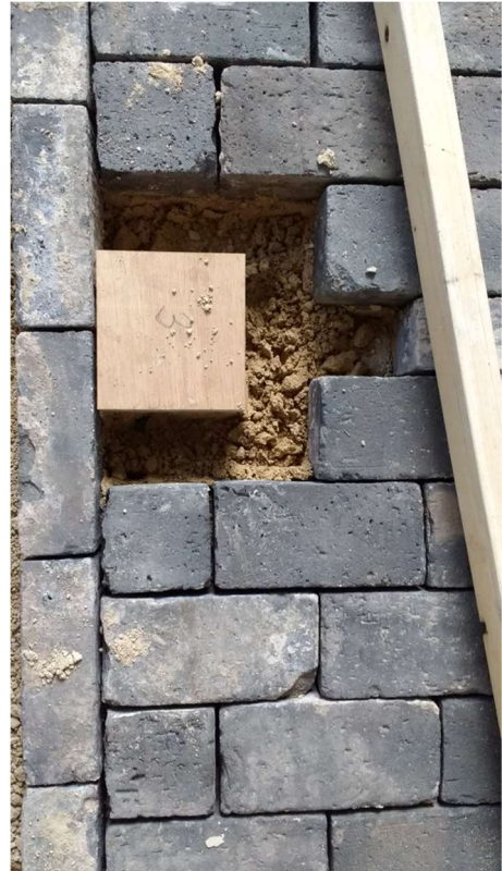
Figure 9: Relaid brick floor with timber inserts above original timber posts discovered during excavation
