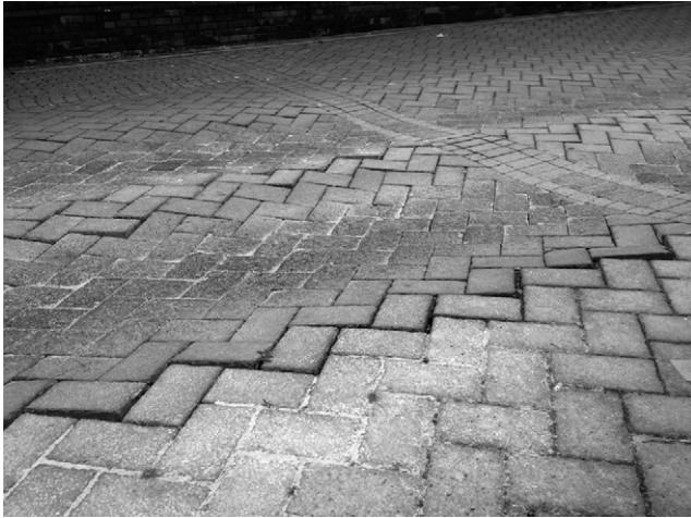
Figure 10. Sunk paving at UK site
