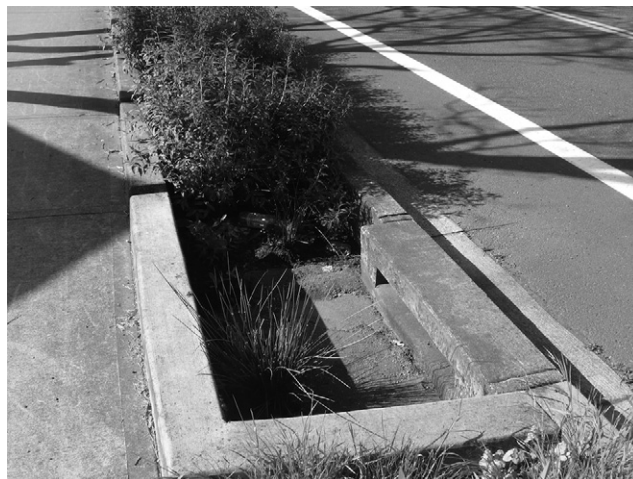
Figure 8. Bioswale inlets in the USA
