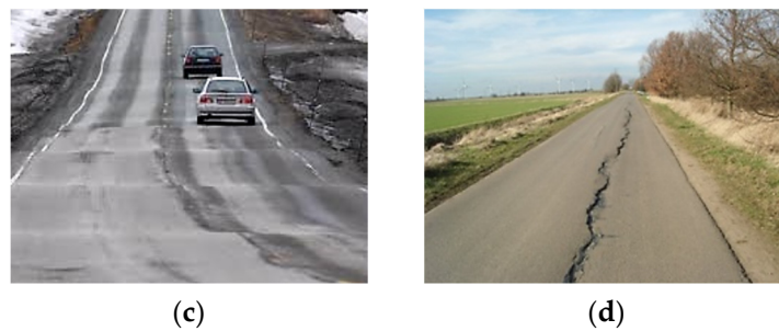
Figure 2. (a) Typical wet expansive soil [14]; (b) typical dry expansive soil [15]; (c) uplifting of flexible pavement due to expansive soil [16]; (d) typical longitudinal crack developed on pavements over expansive clays [17].
