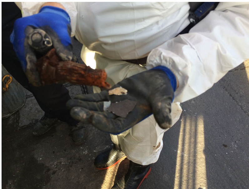
Figure 3. Deterioration: one of the thousands of bolts used to hold the tunnel under the River Avon together.
