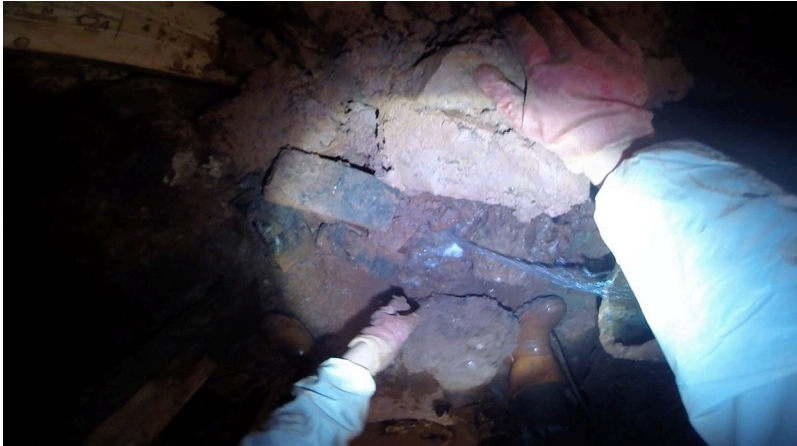
Figure 1. Invisible yet proximate: a miner clearing earth at a broken sewer underneath a street in Clifton, Bristol. Notice the waste water flowing into the tunnel from the pipe on the right.
