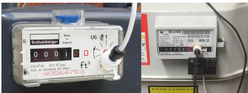
Figure 7 Optical and Magnetic detectors fitted on gas meters
