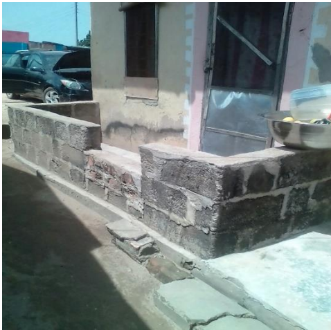
a) A concrete wall constructed to prevent flood from entering the house
