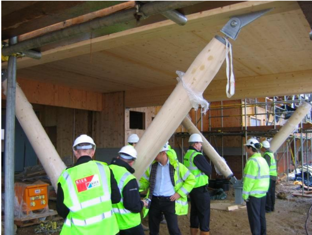
Figure 3. St Augustine School under construction; there were frequent visitors to the site to see the innovative CLT system being installed (photo credit: Alice Moncaster)
