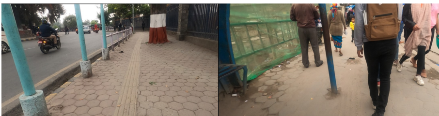
Figure 2. Trees and poles on the pavement causing obstructions—an excerpt taken from the video of P3, vision-impaired.
