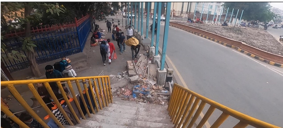
Figure 1. Construction materials piled up on the pavement blocking the stairs—an excerpt taken from the video of P4, vision-impaired.
