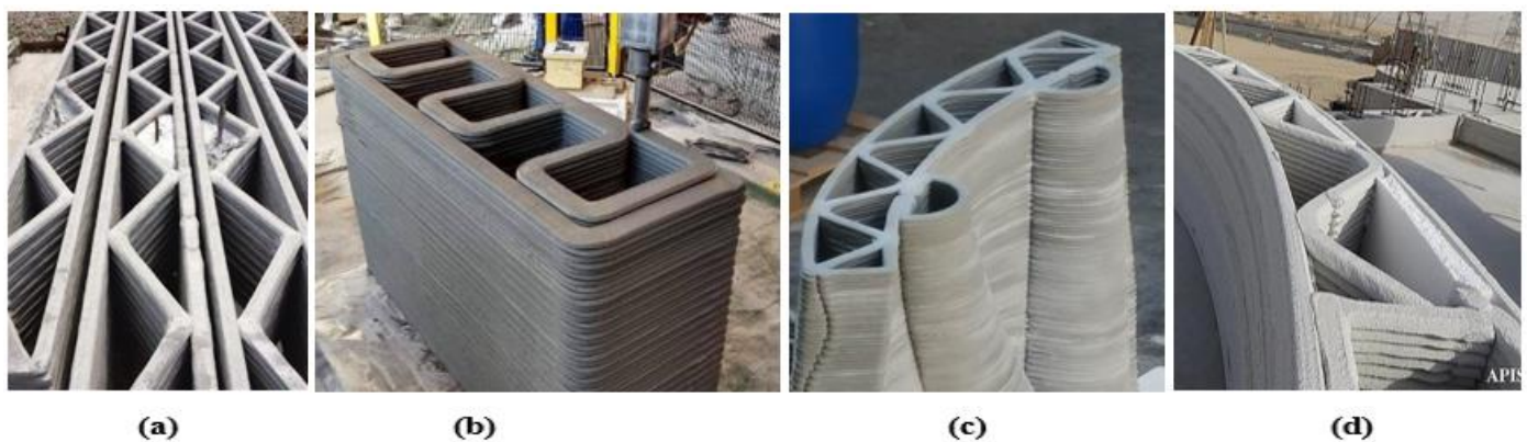
Figure 1. Examples of 3DPC wall panels with different cross-sectional arrangements: (a) triangular-shaped [25]; (b) lattice-shaped 3DPC wall by ETESIAS [26]; (c) sinusoidal-shaped 3DPC wall by Gosselin et al. [27]; (d) sinusoidal shaped, from the world's largest 3DPC building in Dubai [28].
