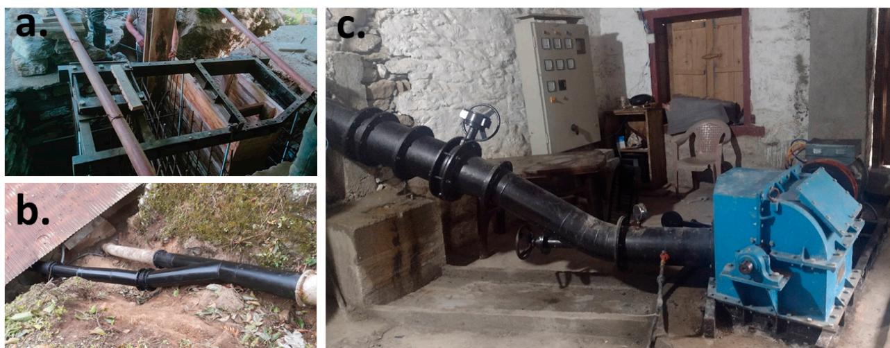
Figure 7. Site works for the renovation, (a) installed y-section of penstock pipe, (b) cementing of new turbine frame, (c) installed Turgo turbine in the powerhouse.
