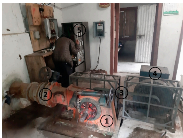
Figure 5. Inside of the powerhouse at Mangmaya Khola I including turbine (1), inlet valve (2), belt drive transmission (3), generator (4) and control panel (5).
