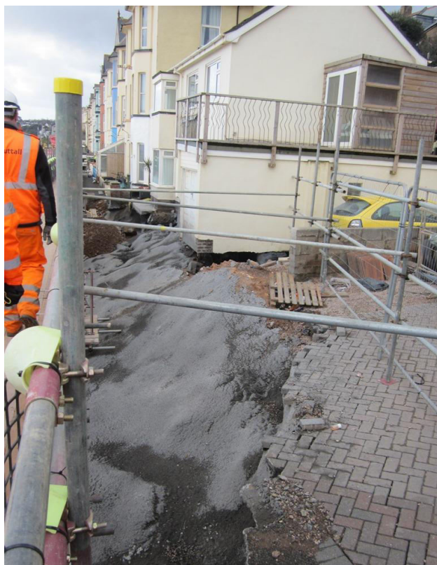
Figure 9. Pictures of the damage occurred on the railway line at Dawlish in February 2014
