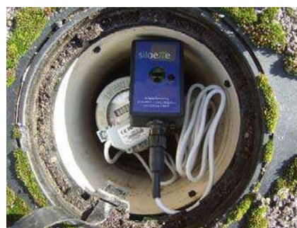
Fig.1. Siloette logger attached to water meter
