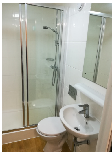
Figure 3. Shower/WC room. Used with permission of the creator.
