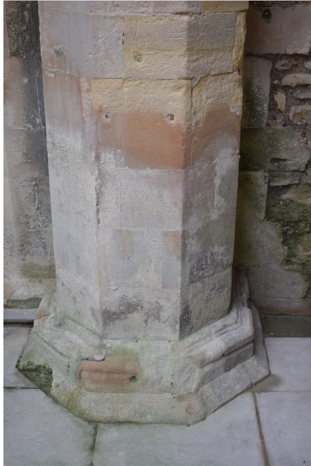
Figure 3.5: An image showing a likely efflorescence at the base of a column in the Royal Garrison Church. The location of the weathering front suggests that this is the result of capillary rise of saline groundwater.
