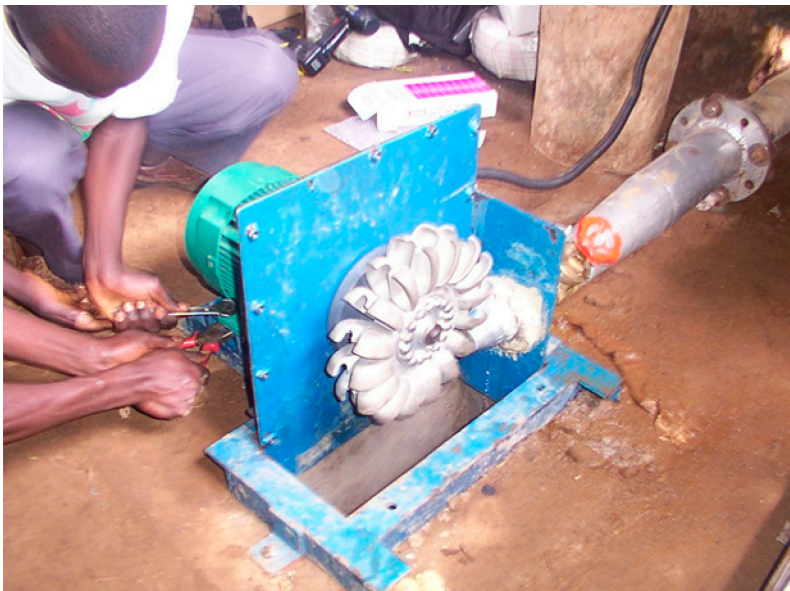
Figure 20. Pico Power Pack with casing removed (Photo credit: Phil Maher, Hydromatch Ltd.).
