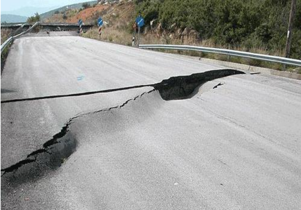
Figure 1.7: Differential settlement due to expansive subgrade (U.S. Department of Transport, 2020)
