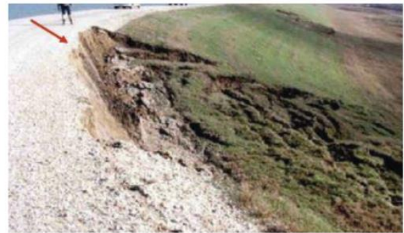
Fig. 5. Slope failure of embankment caused by expansive soil (Jalal et al., 2020).
