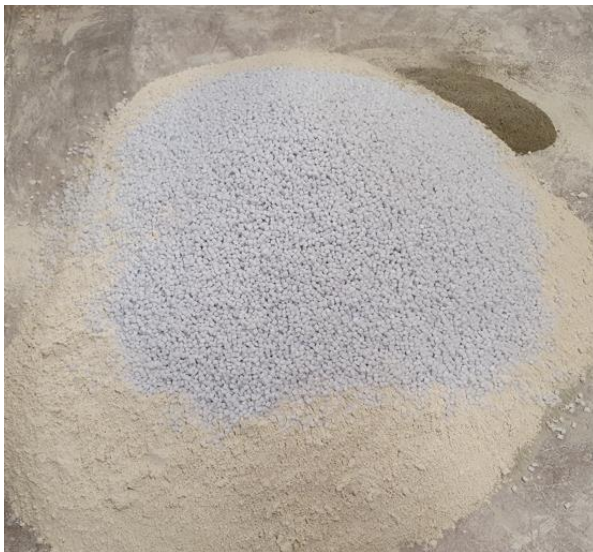
Recycled plastic pellets and other binders added to subgrade material during the mixing process
