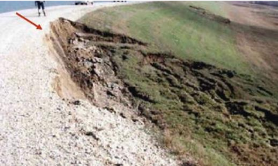
Figure 1.8: Slope failure of embankment caused by expansive soil (Jalal et al. , 2020)
