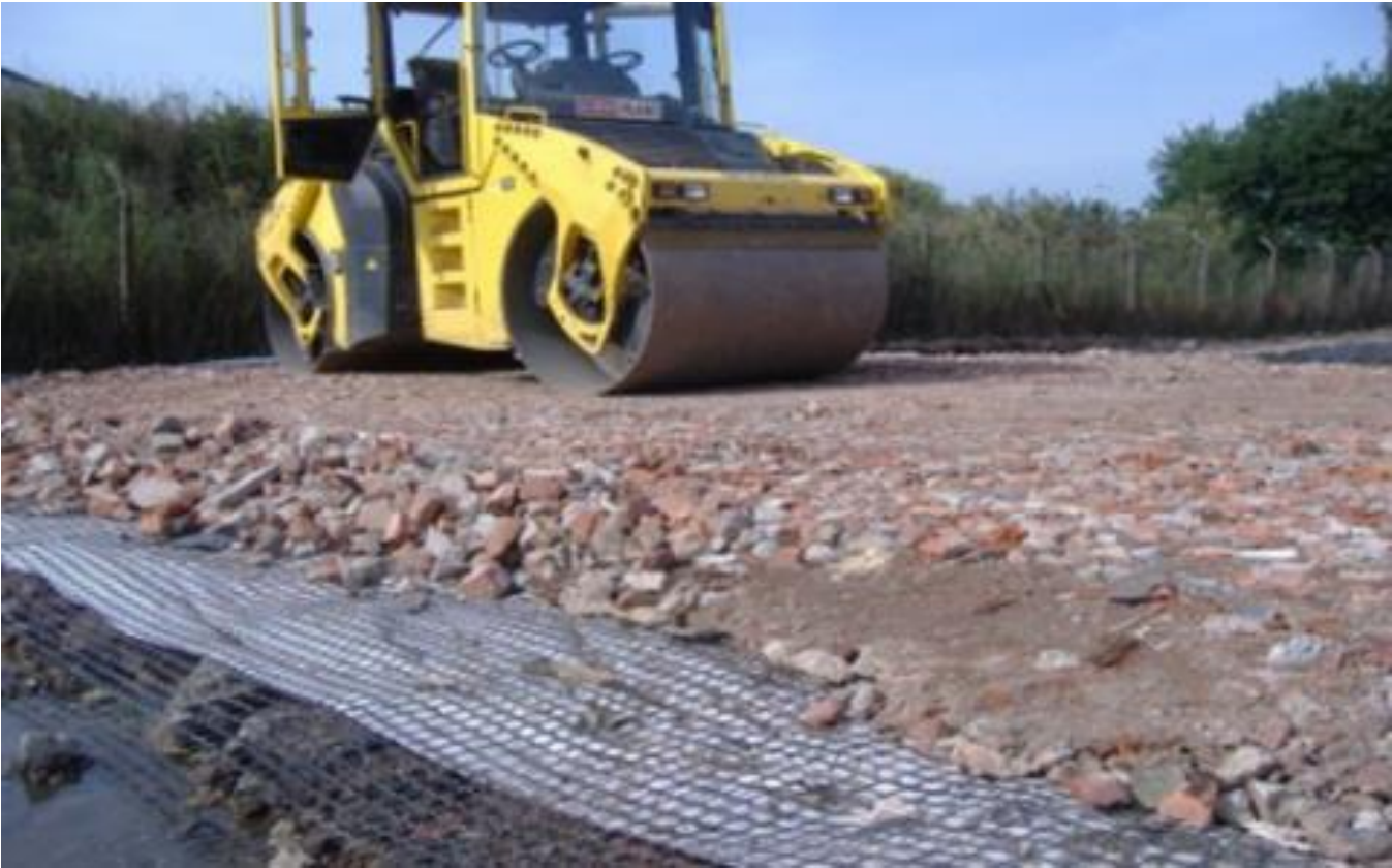
Figure 2.12: Construction and demolition waste, geogrid and textile used in road construction (ABG Geosynthetics, 2020)
