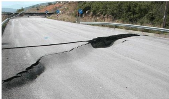
Fig. 2. Road pavement defect (U.S. Department of Transport).
