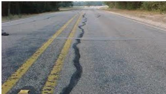
Fig. 3. Typical longitudinal crack developed on pavements over expansive clays (Zornberg and Gupta, 2015).
