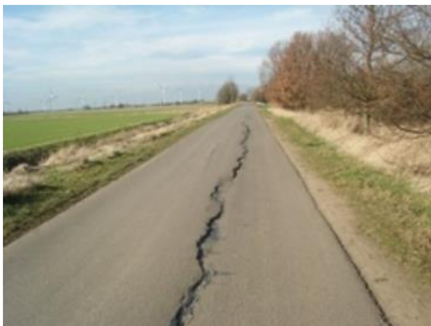
Figure 1.6:Typical longitudinal crack on road pavement (The geological society, 2012)
