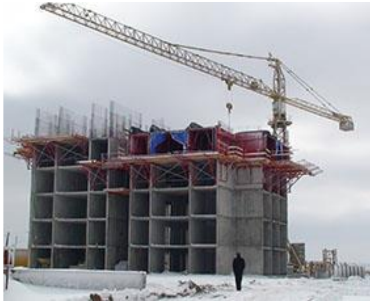
Fig. 1 Concrete casting of box-type buildings (photo taken by the authors from a project)
